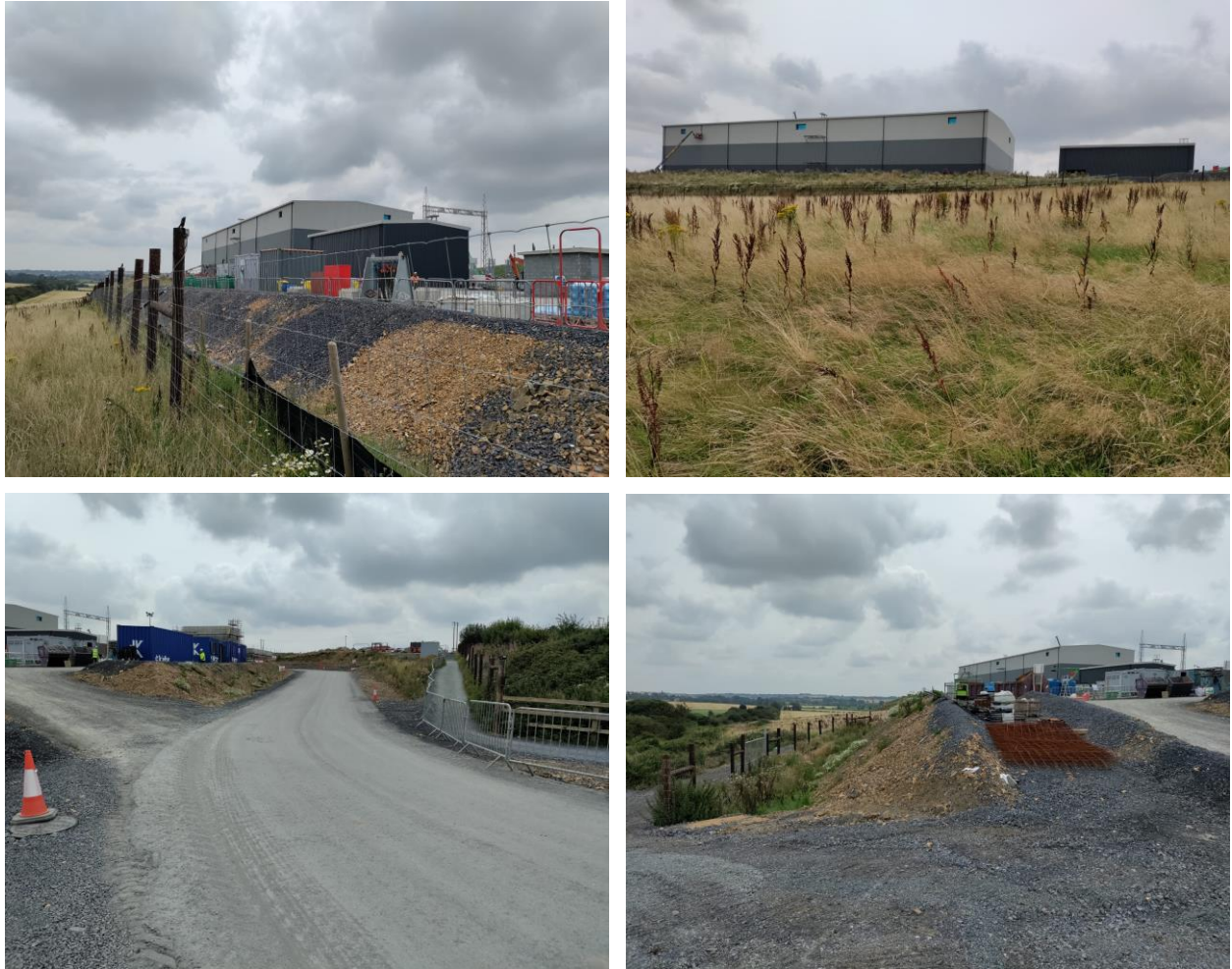
Figure 9 – Greenlink Converter Station (under construction) – clockwise from left to right – converter station from southern boundary of Site; converter station from centre of Site; converter station access road; access road to Site
